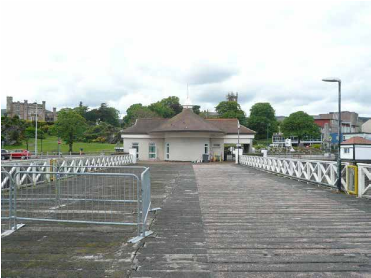
Souther Arm of Pier – May 2014. Note bitumen covering to decking boards, irregular gaps between boards, joints between boards run along the centre and uneven surface.
