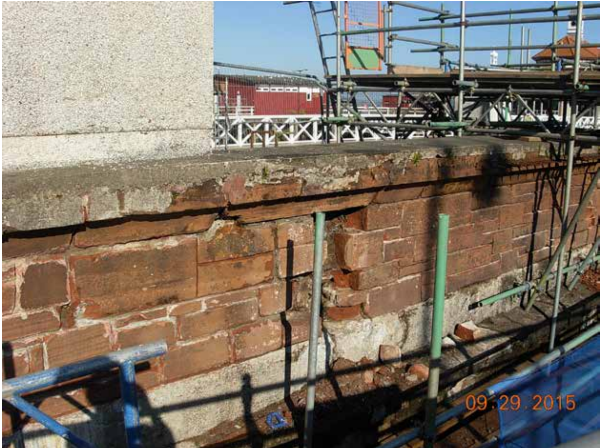
Retaining Wall to Harbourmasters Building – Note condition of stonework and pointing
