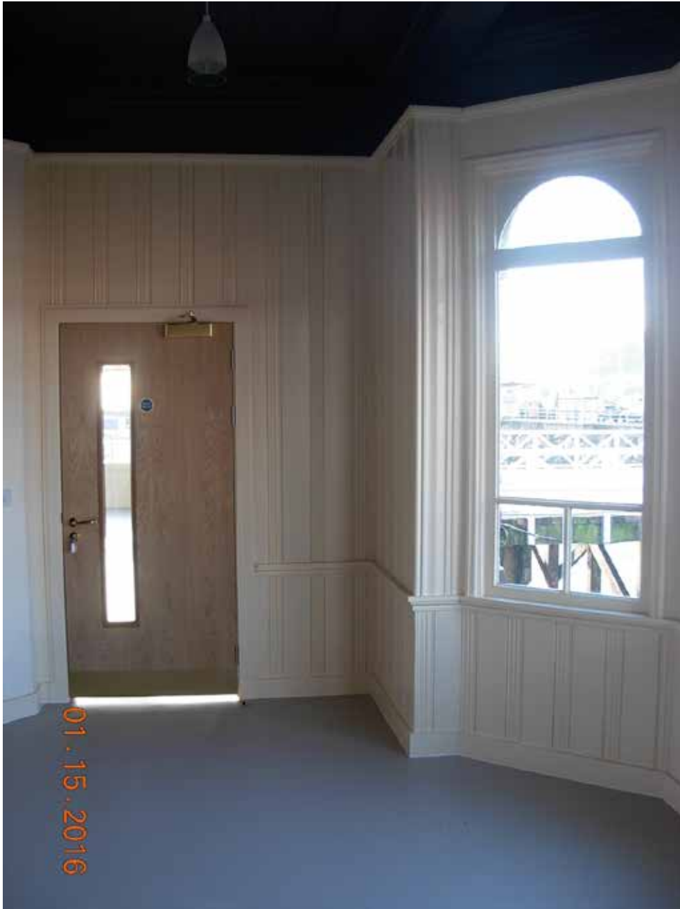
Ground Floor Entrance Lobby: tea-prep facility on the right hand side and new access into the First Class Waiting Room
