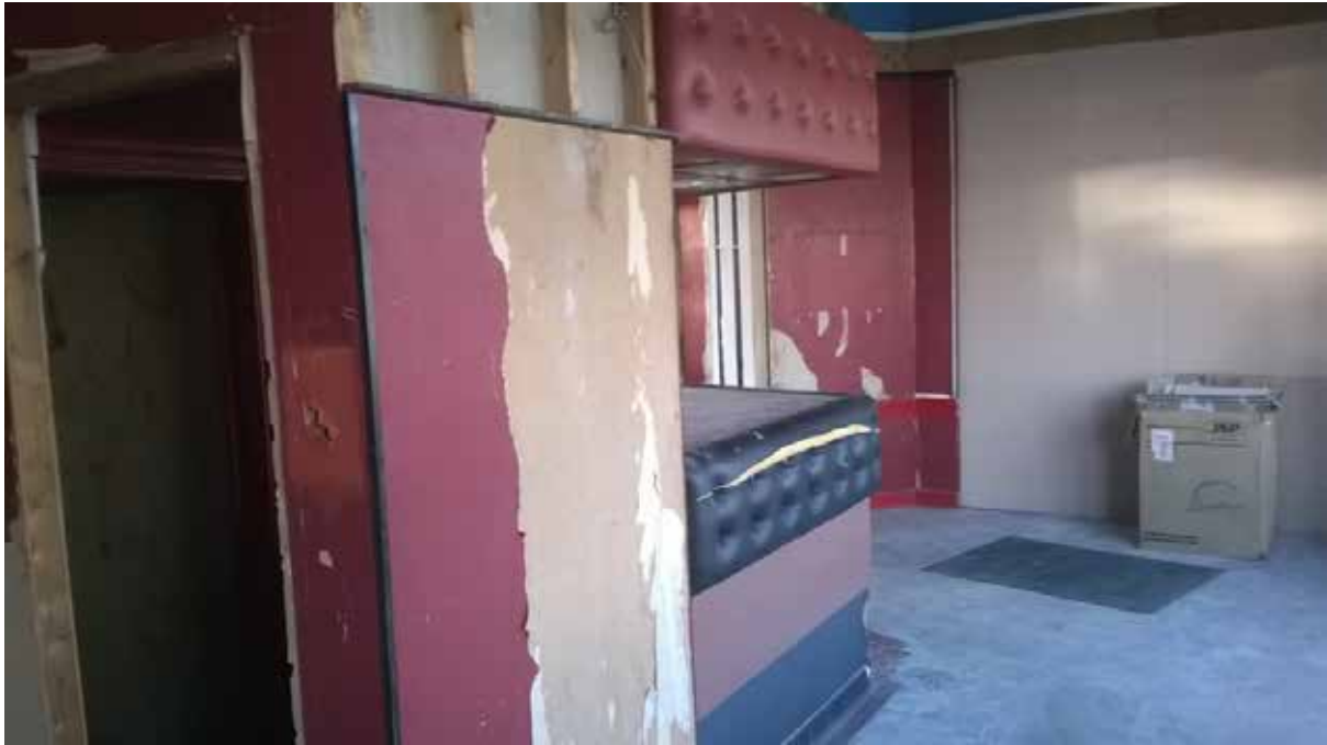
Ground Floor Entrance Lobby – November 2014. Area in the background has been refurbished to provide tea-prep facility and access into the First Class Waiting Room. Area in the foreground has been refurbished to provide ladies and gents toilets and cleaners store/cupboard and access corridor between First Class and Third Class Waiting Rooms
