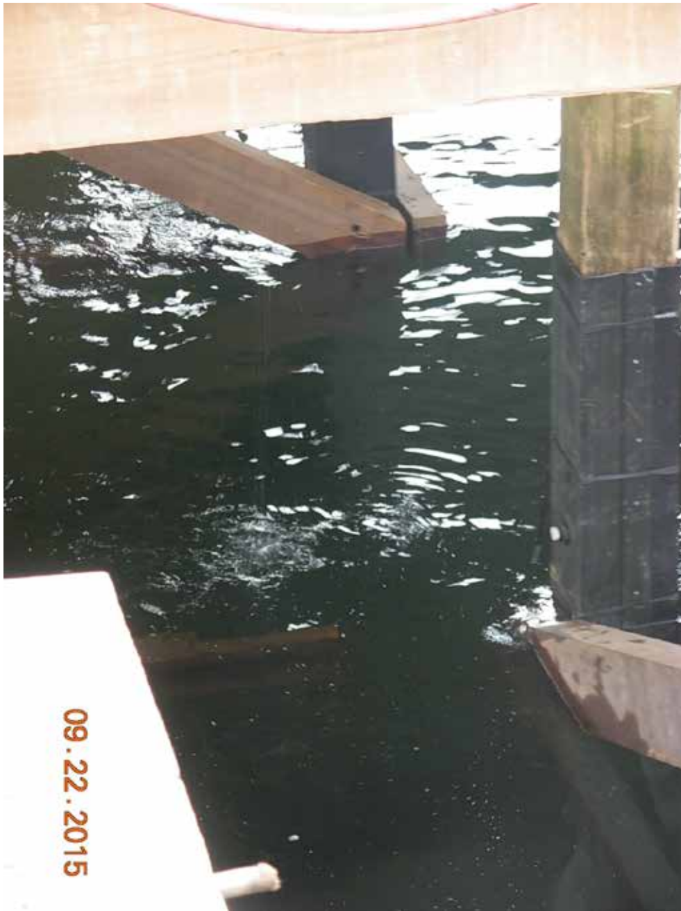
Structure of Pier – an example of the epoxy encapsulation system to an existing timber column. These works were confined to the areas of the structure underneath the Waiting Room building where it would not have been possible to replace the timber column.
