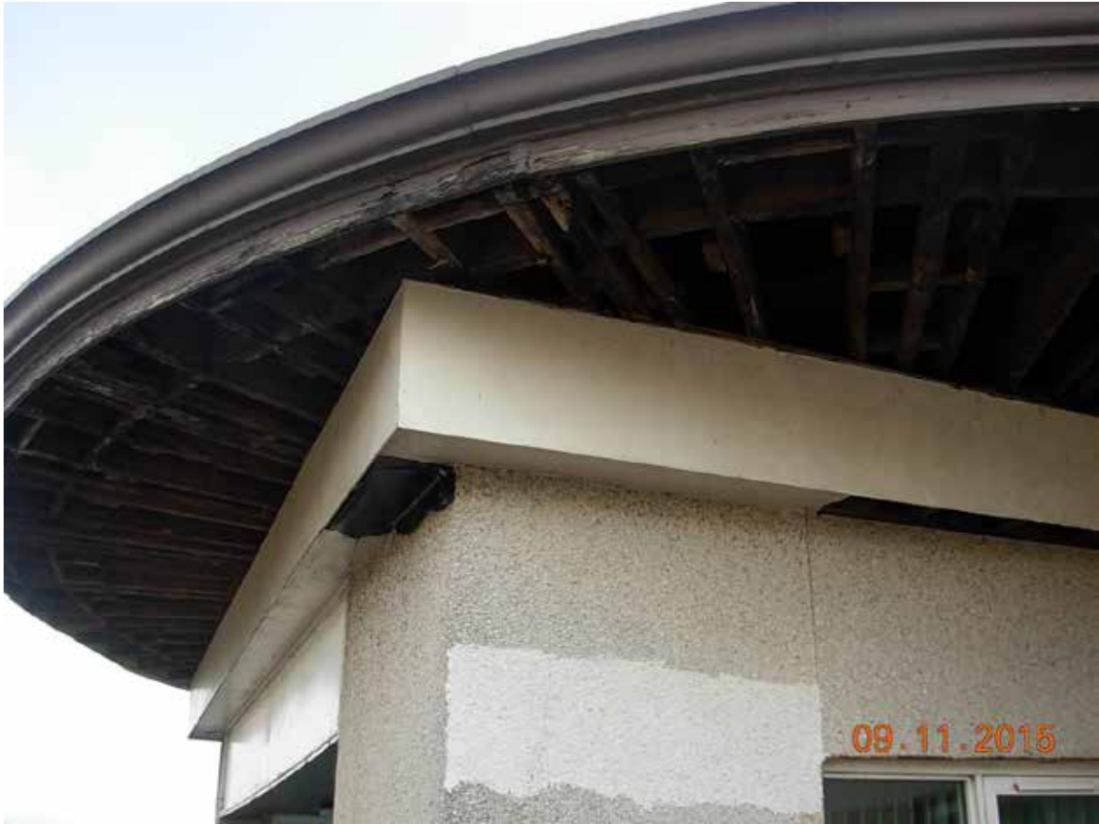
Harbourmasters Roof – Note rotten joists, soffits and fascias which has been caused by internal downpipes leaking and gutters having corroded.
