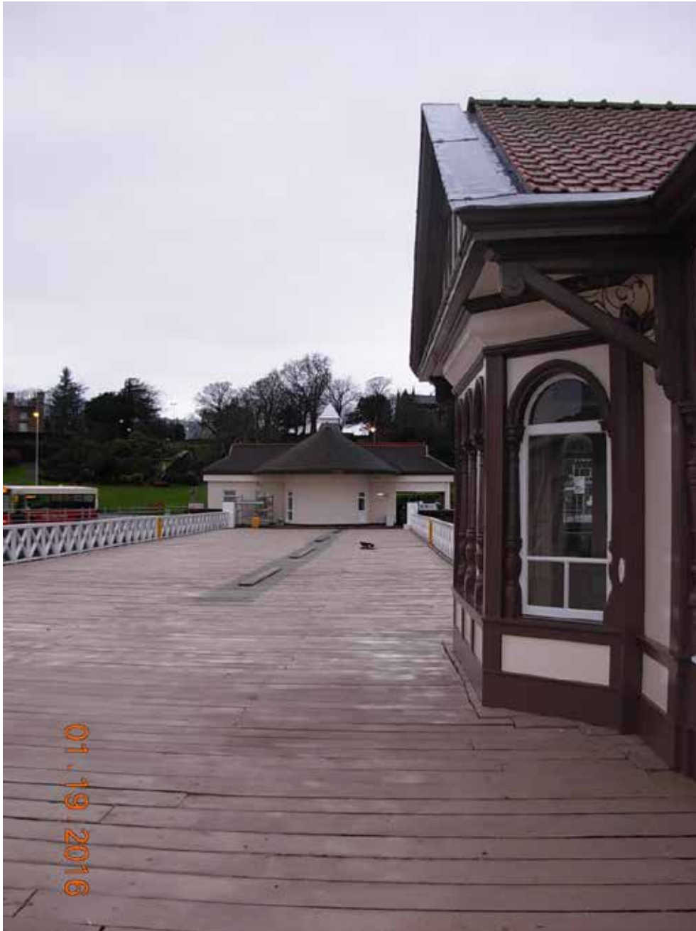
Southern Arm of Pier – January 2016. Note the gaps between the decking boards have been closed up, joints between boards have been staggered, surface is now more level, antislip treatment has been applied across the full width of the deck and handrails have been refurbished.
